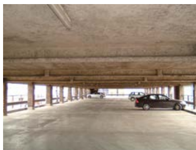
Figure 7 Sprayed limpet on car park roof
