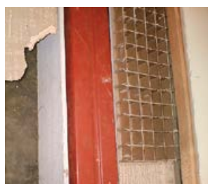
Figure 21 AIB column fire protection in CLASP building
