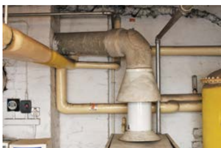
Figure 34 Asbestos cement boiler flue
