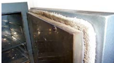
Figure 26 Asbestos rope seal on drying oven
