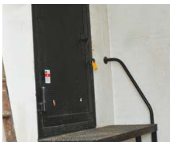
Figure 45 'Durasteel' composite steel and asbestos fire door
