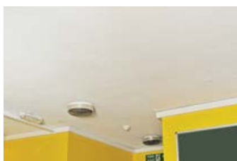
Figure 36 Asbestos textured coating on ceiling
