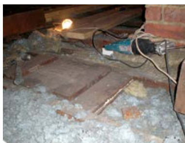
Figure 6 Loose asbestos used as loft insulation
