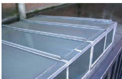
Figure 31 Chrysotile string on skylights
