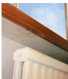
Figure 20 AIB panel between radiator and window
