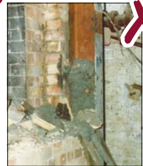
Sprayed asbestos (limpet)
