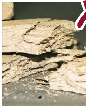
Broken asbestos insulating board
