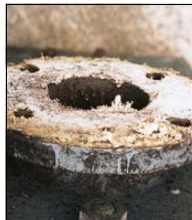
Gasket material left on a pipe flange
