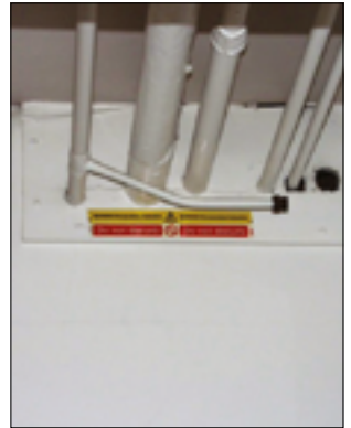
Don't assume there will always be warning signs. There could be undiscovered asbestos in buildings you work on
