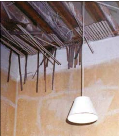
Old lath and plaster ceilings are often covered in textured coating to hide imperfections
